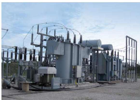
▲ Transformer stations are just one asset to be managed by utilities.
