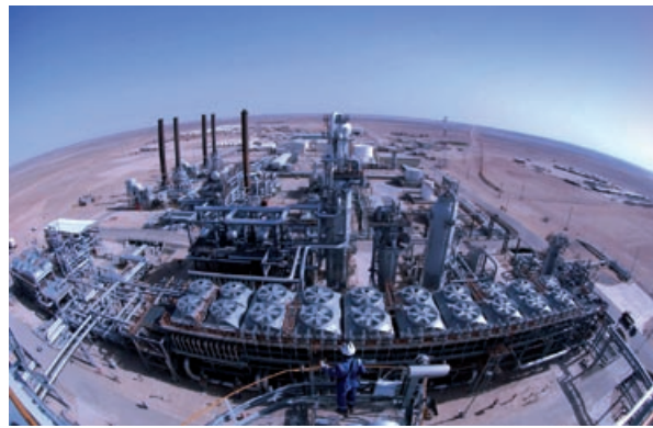
▲ CO 2 storage at the In Salah natural gas production facility (Algeria).
