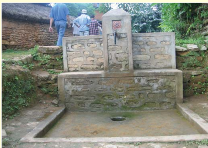
Water distribution tap of community managed water pumping system
