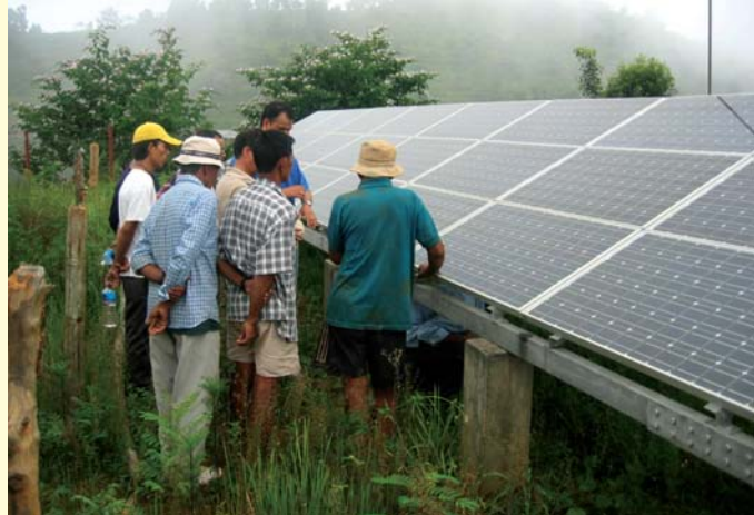
Community managed solar water pumping system
