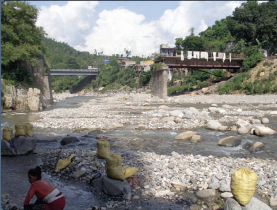
Figure 3: Impact of flash flood due to the 1993 cloudburst event in the headwater area of Malekhu khola in the Mid Zone of Nepal: half of a bridge on the Prithvi Highway in the plains was washed away. A new bridge can be seen in the background
