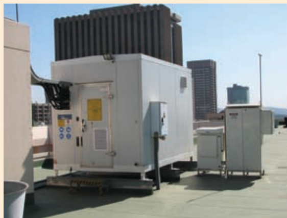
GenCore Fuel Cell installation at the Vodacom Skinner Street site in South Africa
