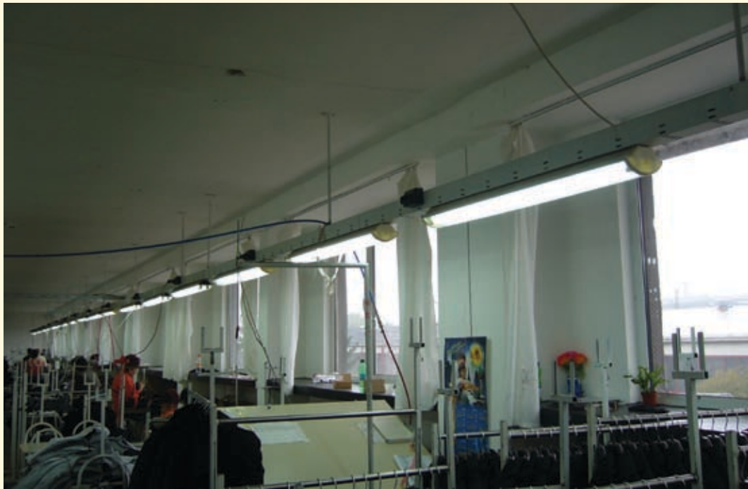
The BEEF project brings efficient lighting and heating for an apparel factory in Plevna, Bulgaria
